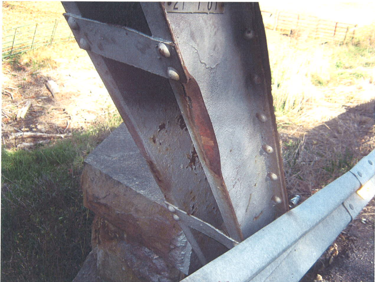
LOG C21-1.00 – L0U1 NORTH TRUSS EAST END – NOTE DAMAGE
