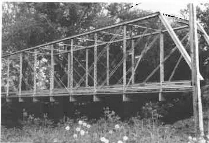
Tension members on this 140-foot Whipple truss bridge are proportioned according to a formula devised after the Civil War by a prominent civil engineer from St. Louis, C. Charles Shaler. Diagonals increase in section towards the end, while the lower chord eyebars are largest in the center panels.
